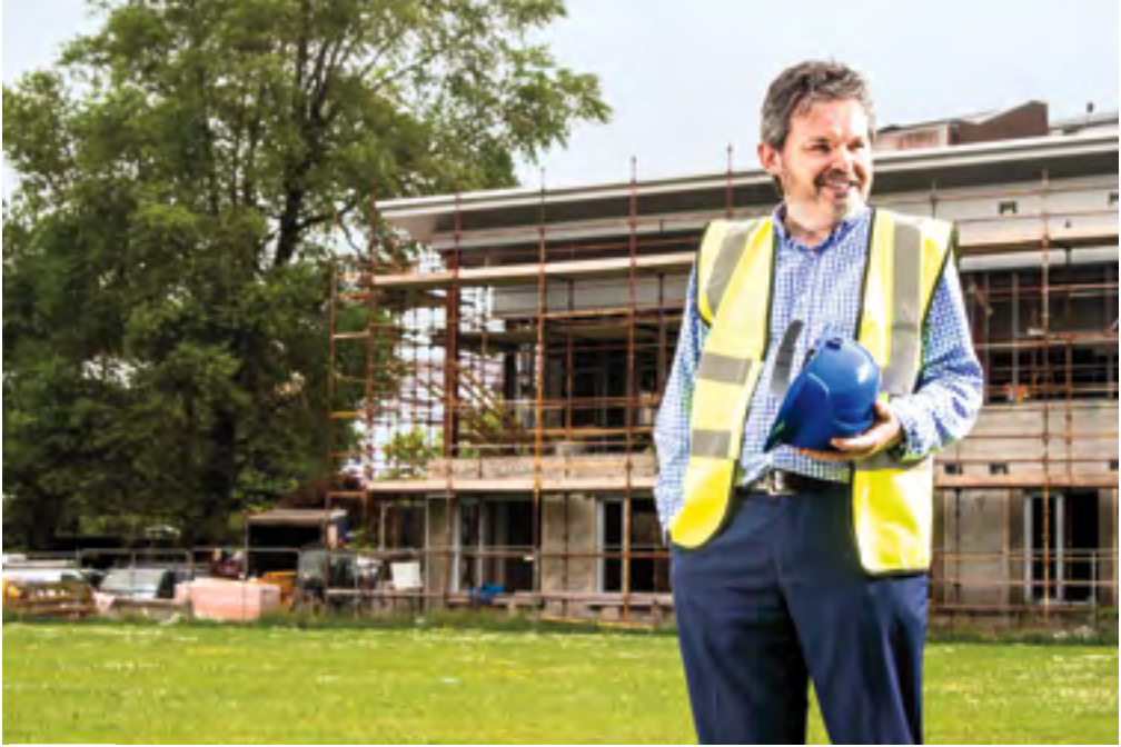
Lauri McCusker, director of Fermanagh Trust, checks out a school building under construction.
