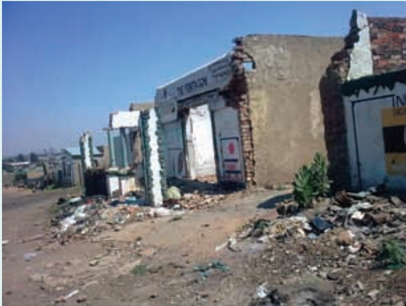
Figure 4: A vandalised structure belonging to a foreigner
